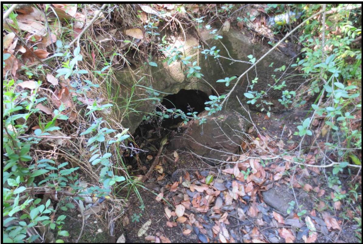
Plate 8 View showing build-up of debris on upstream side of culvert
