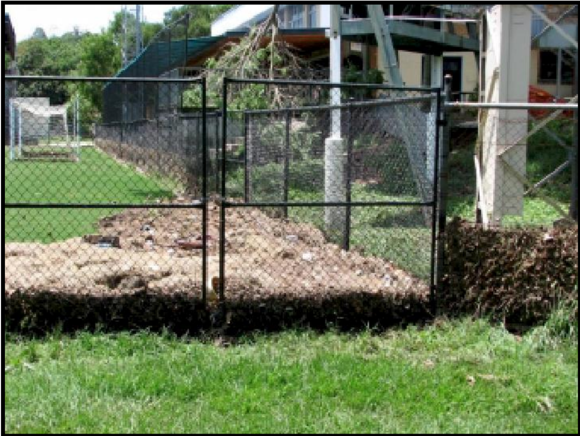
Plate 9 Example of wire mesh fence that has collected debris during a flood, which may cause blockage of flow paths in urban environments (Engineers Australia, 2009).
