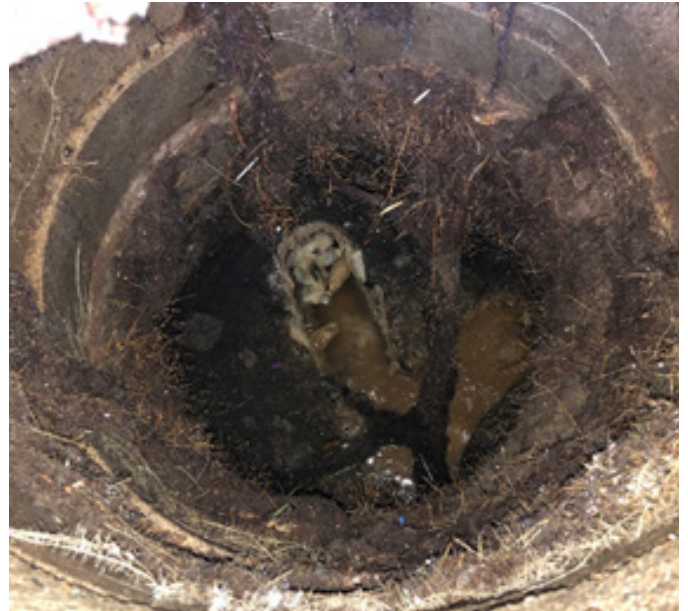
Photo 5: Root intrusion - maintenance hole
