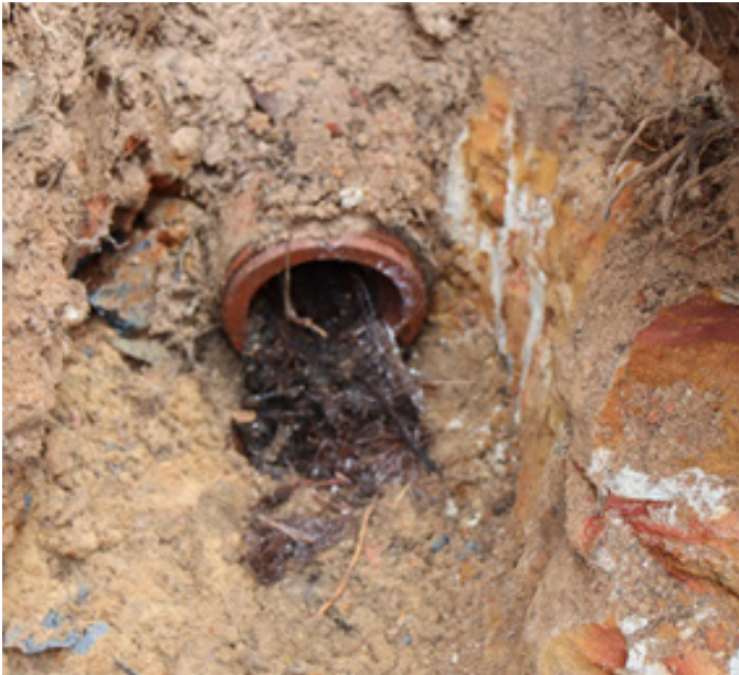
Photo 4: Root intrusion - private sewer pipe
