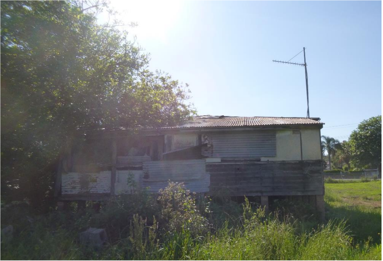
Photograph 3: OI 4 Table 3-1 of Report, abandoned residential dwelling
